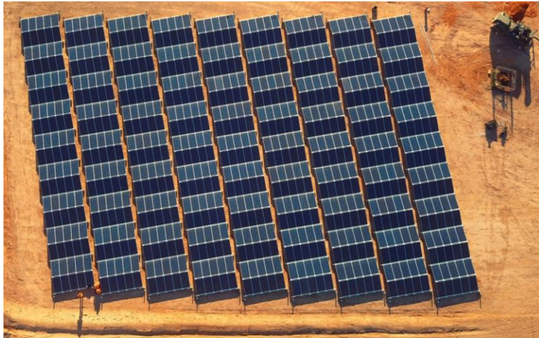
Solar Farm Utilising HVDC Cables
